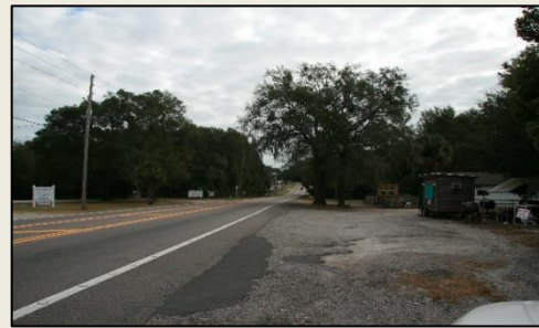
“Lack of sidewalks and street lighting. Deficient parking areas.”
